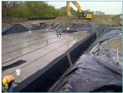
Underground SWM Chamber
